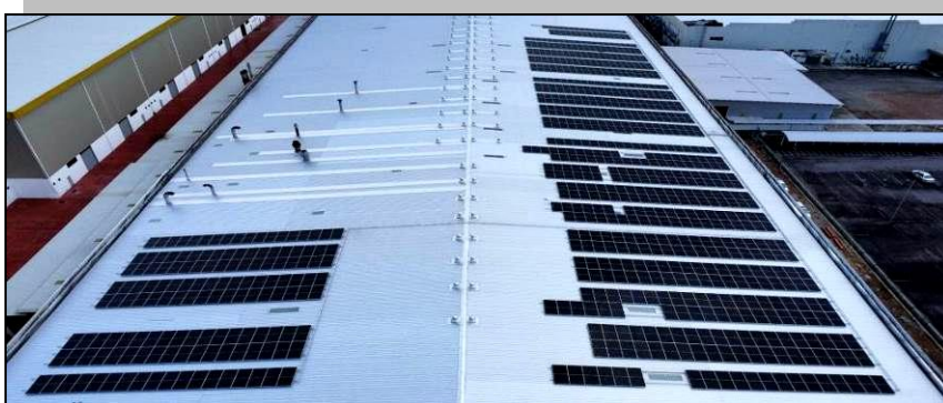
Picture 1: 910 pieces of Jinko solar panels on the factory roof top.
